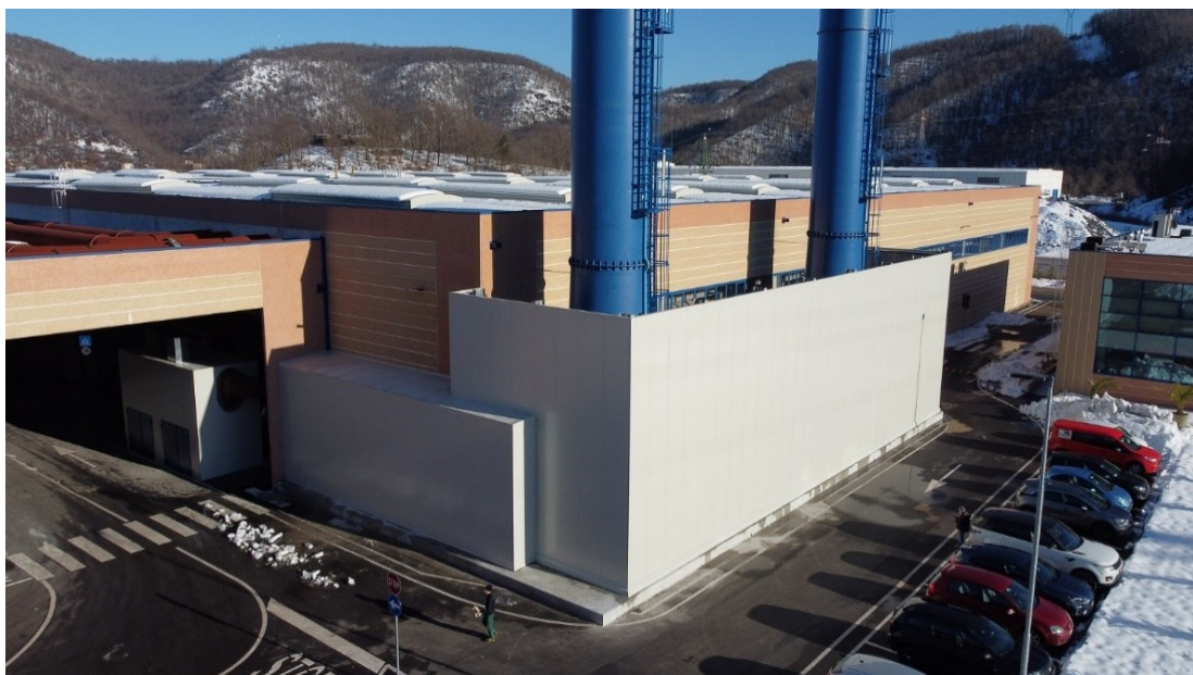
Figure 5 – Sound barrier and fan enclosing – January 2021
